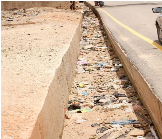
One of the drainages where refuse was dumped
